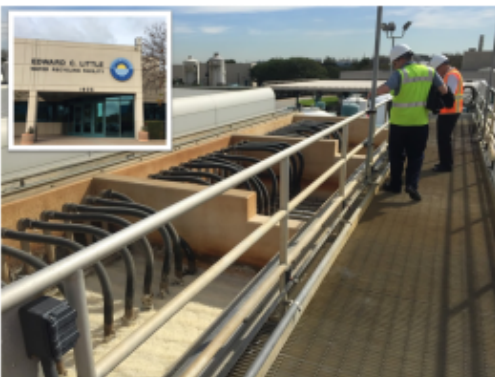
Inset: Edward C. Little WRF; Main: Submerged Membrane Filtration System
